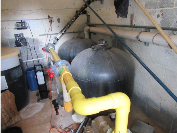
Mechanical pool equipment overview
