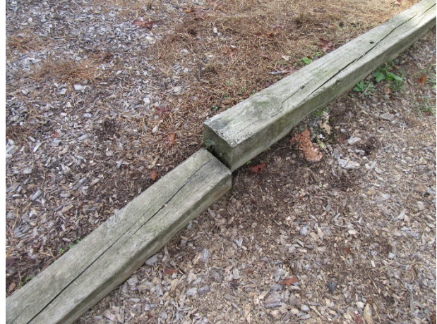
Timber border displacement – Note: Whipple Court
