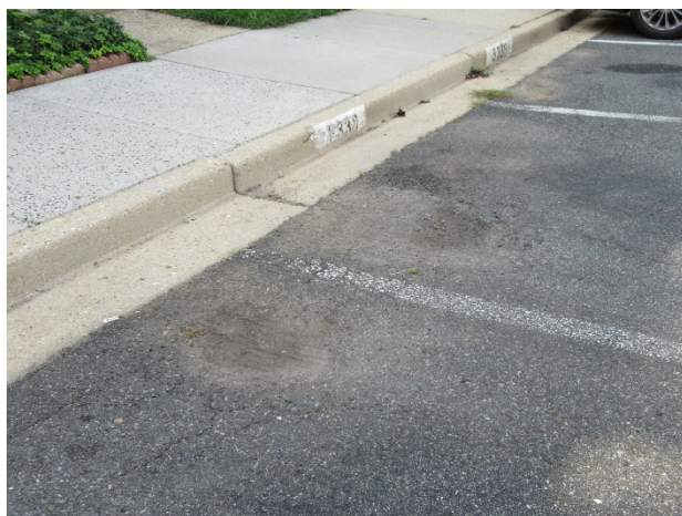
Vehicular fluid stains and rutting – Note: Webley Court
