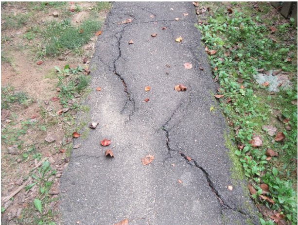
Walking path cracks
