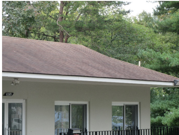
Asphalt shingle roof overview – Note: stains
