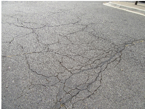
Cracks and previous repairs – Note: Webley Court
