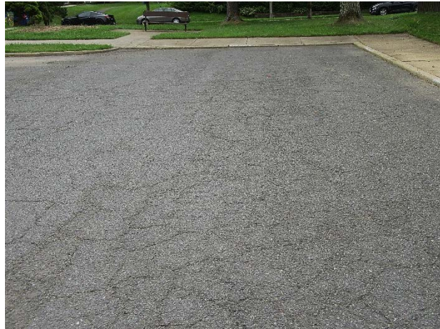
Asphalt pavement overview – Note: extensive cracks at Applegate Court
