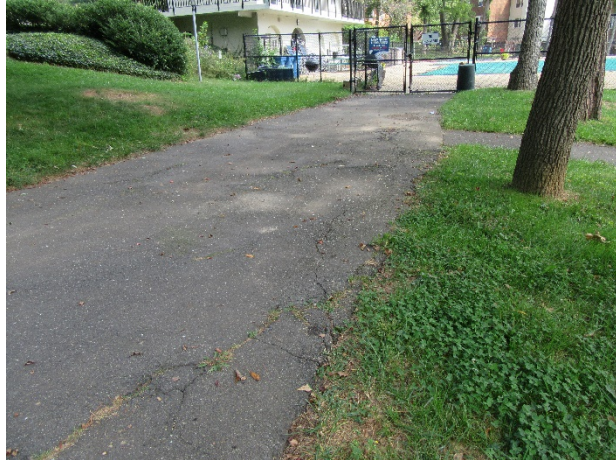
Asphalt pavement pool access drive overview – Note: cracks
