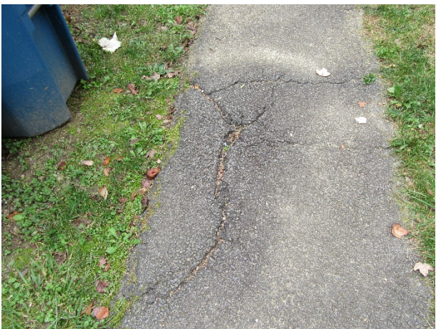
Walking path cracks
