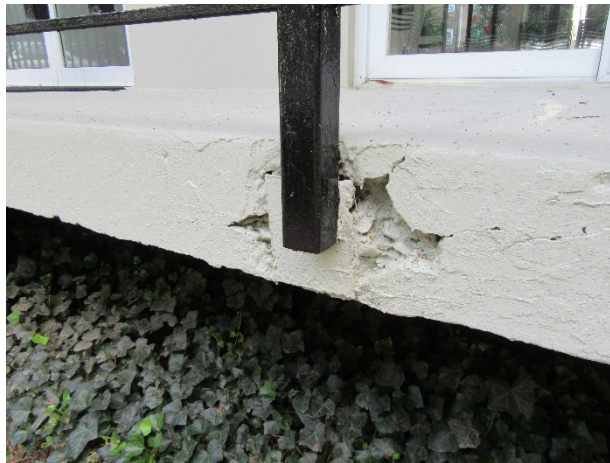
Concrete deck cracks and deterioration
