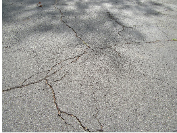
Cracks – Thompson Road
