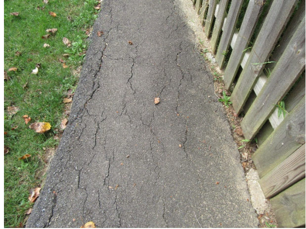
Walking path cracks
