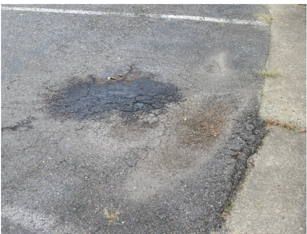
Vehicular fluid stain and rutting – Note: Webley Court
