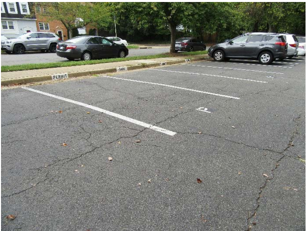
Cracks – Note: Thompson Road
