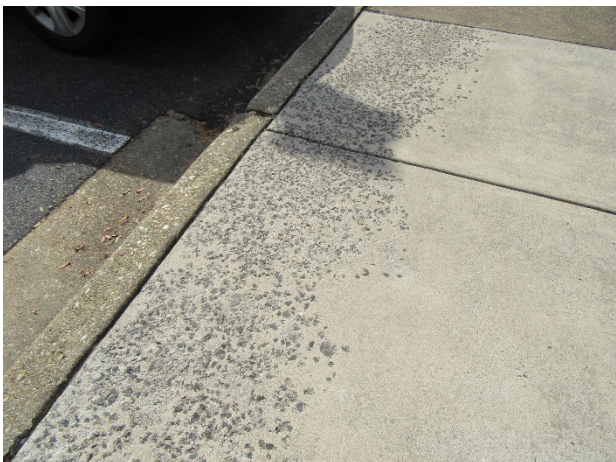
Concrete sidewalk scaling
