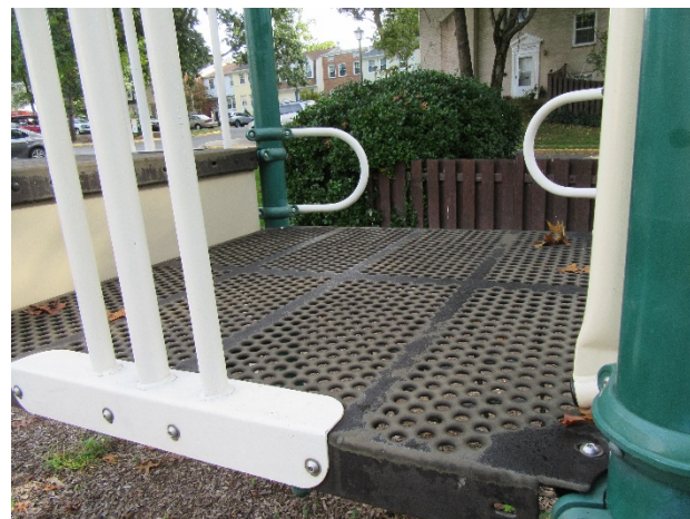
Finish deterioration – Note: Whipple Court
