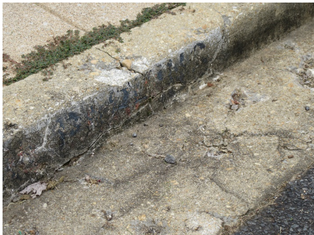
Cracks and deteriorated concrete
