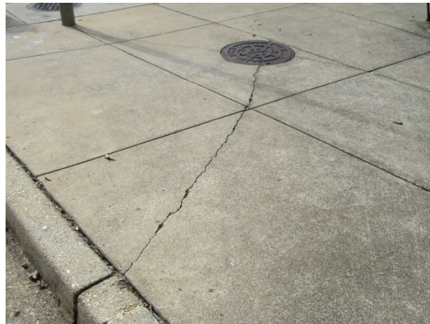
Concrete sidewalk crack
