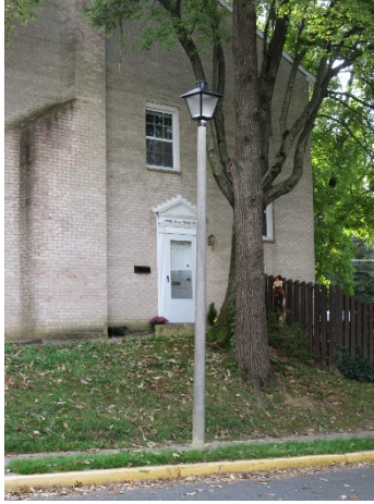
Light pole and fixture overview
