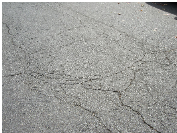
Cracks – Note: Glastonbury Court
