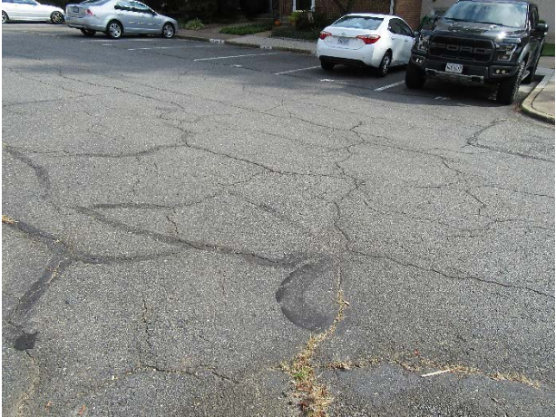
Cracks and previous repairs – Note: Webley Court
