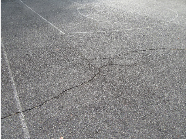
Basketball court cracks
