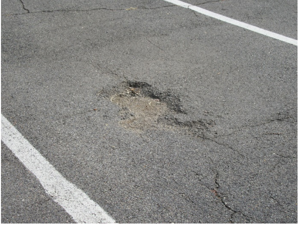
Pothole and cracks – Contessa Court
