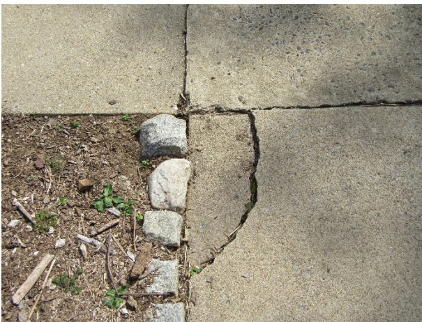
Concrete sidewalk crack
