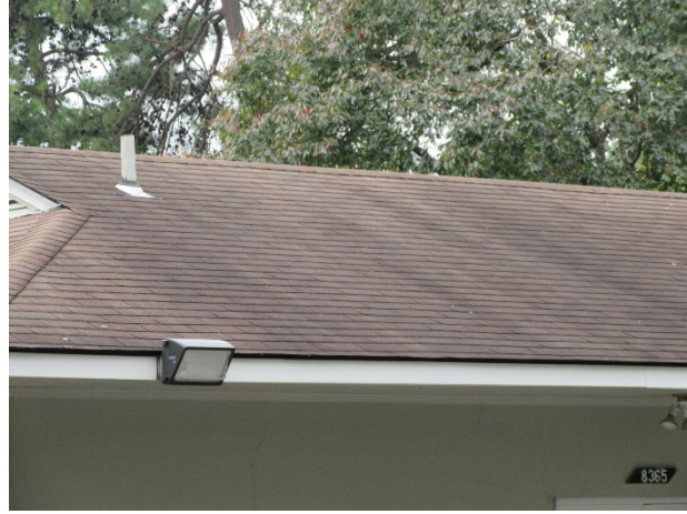
Asphalt shingle roof overview – Note: stains
