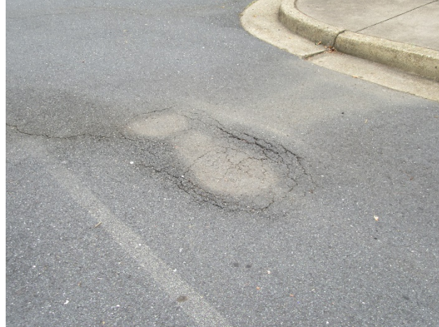
Rutting – Note: Viscount Court
