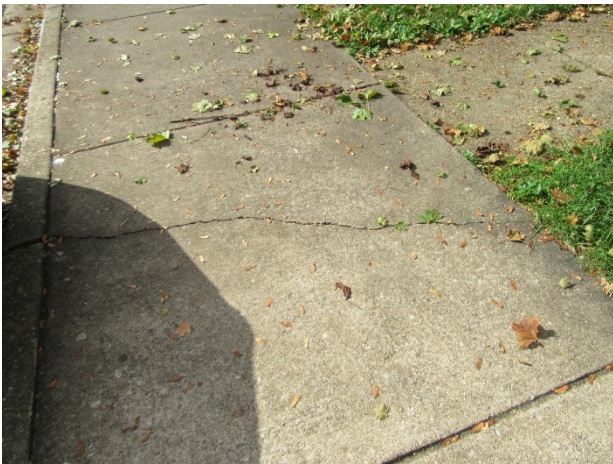
Concrete sidewalk crack
