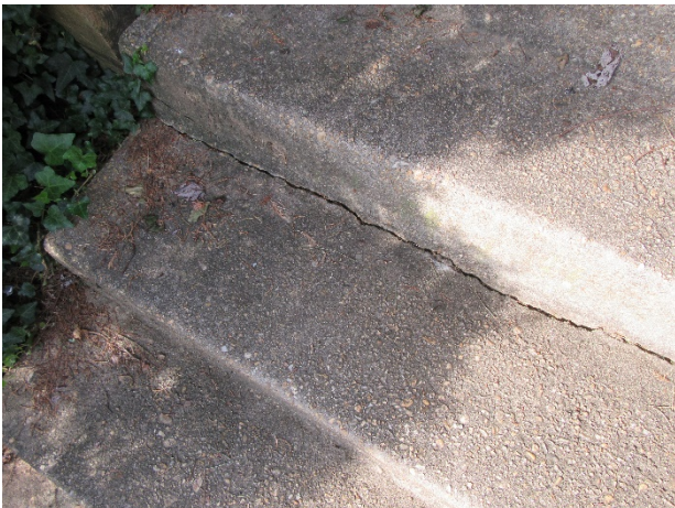
Concrete stair crack
