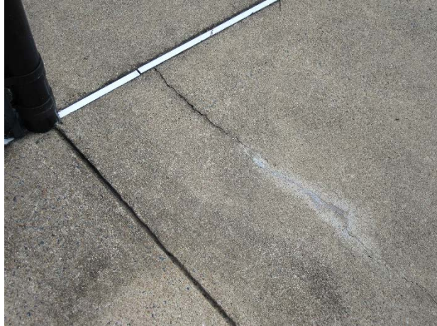
Concrete crack and previous repair
