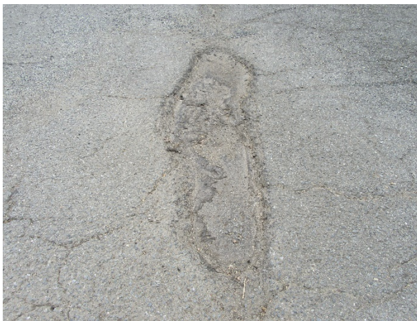
Pothole and cracks – Note: Applegate Court
