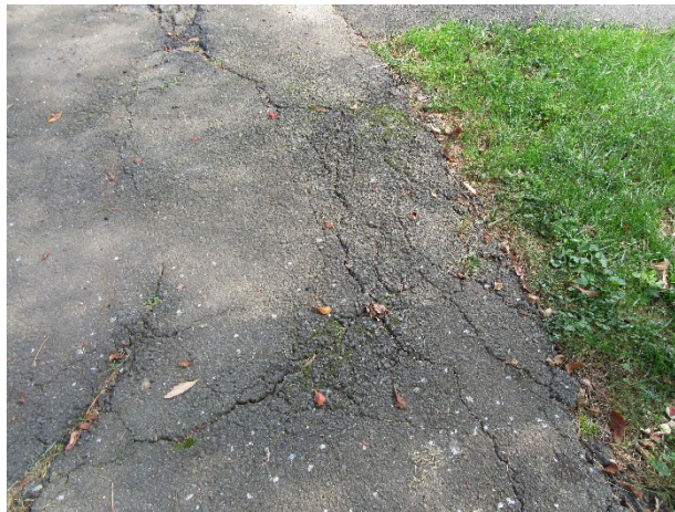
Pool access drive cracks
